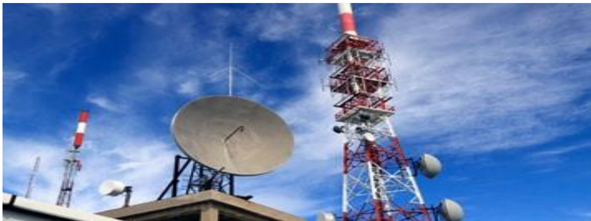
Figure 1: Telecommunication base station site
